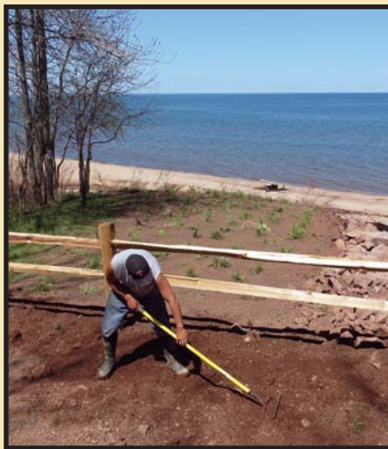
Dan Wiggins Jr. puts finishing touches on the split rail fence at Waverly Beach
