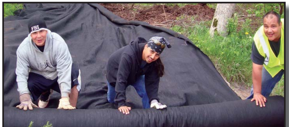
Evan Rosin, Shane Cadotte, and Ben Connors help roll out the geotextile base of the trail.
